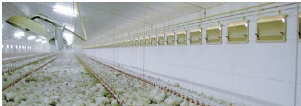
TPI's wall valve, type 3000-VFG. Here in a cross ventilation system in a broiler house.
